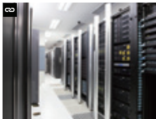
Data center in Yongin
